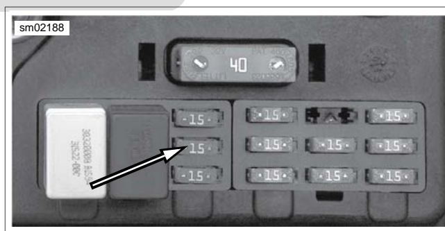
Figure 7-11. Fuel Pump Fuse
