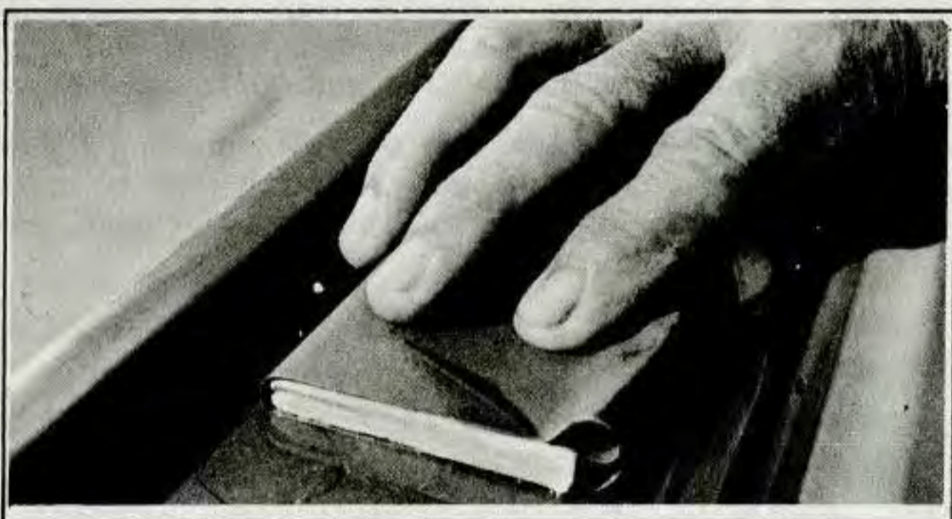
Figure 2J-6. Sanding Patch
